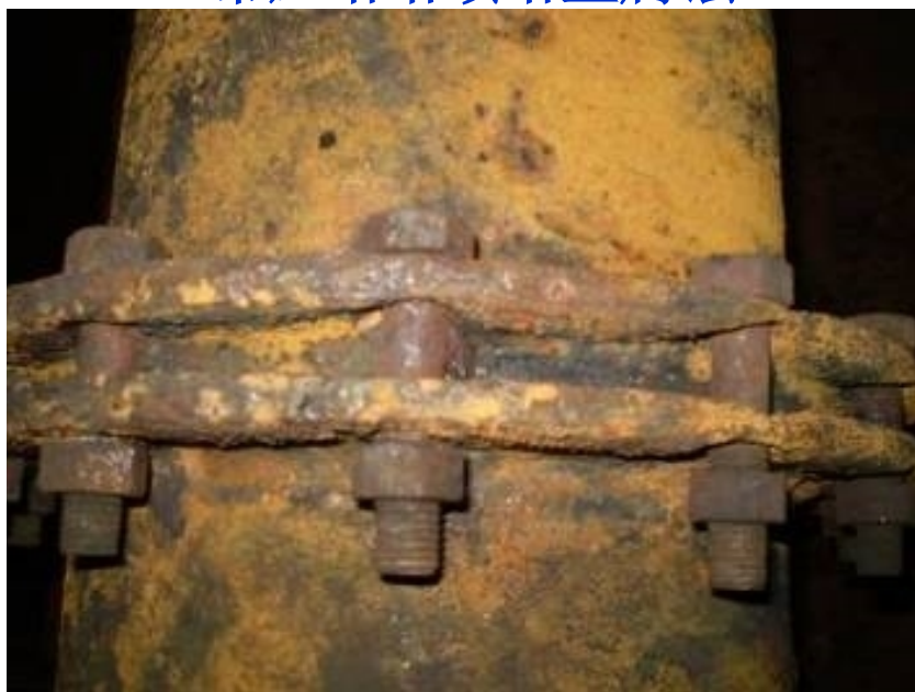
常顶回流管法兰腐蚀减薄
